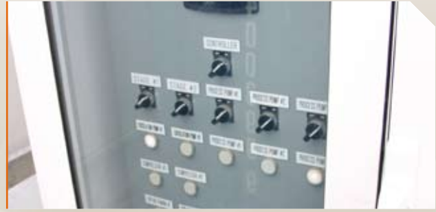
> Panel de control
